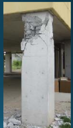
損傷度IVの柱
